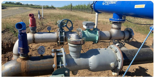
Valve manifold at the pump
